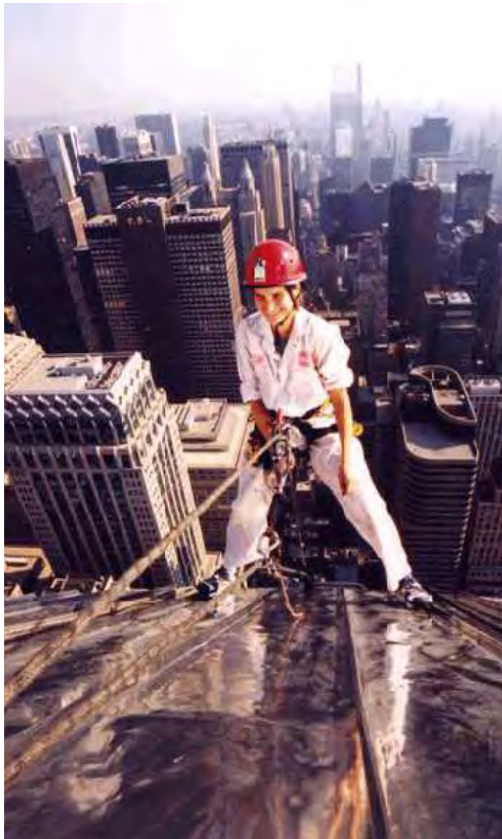
Chrysler Building standing seam water leakage testing Andrea Gaffney BUILDINGS / PROFESSIONAL
