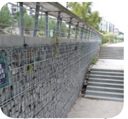
Gabion edges filter and direct stormwater on the site.
