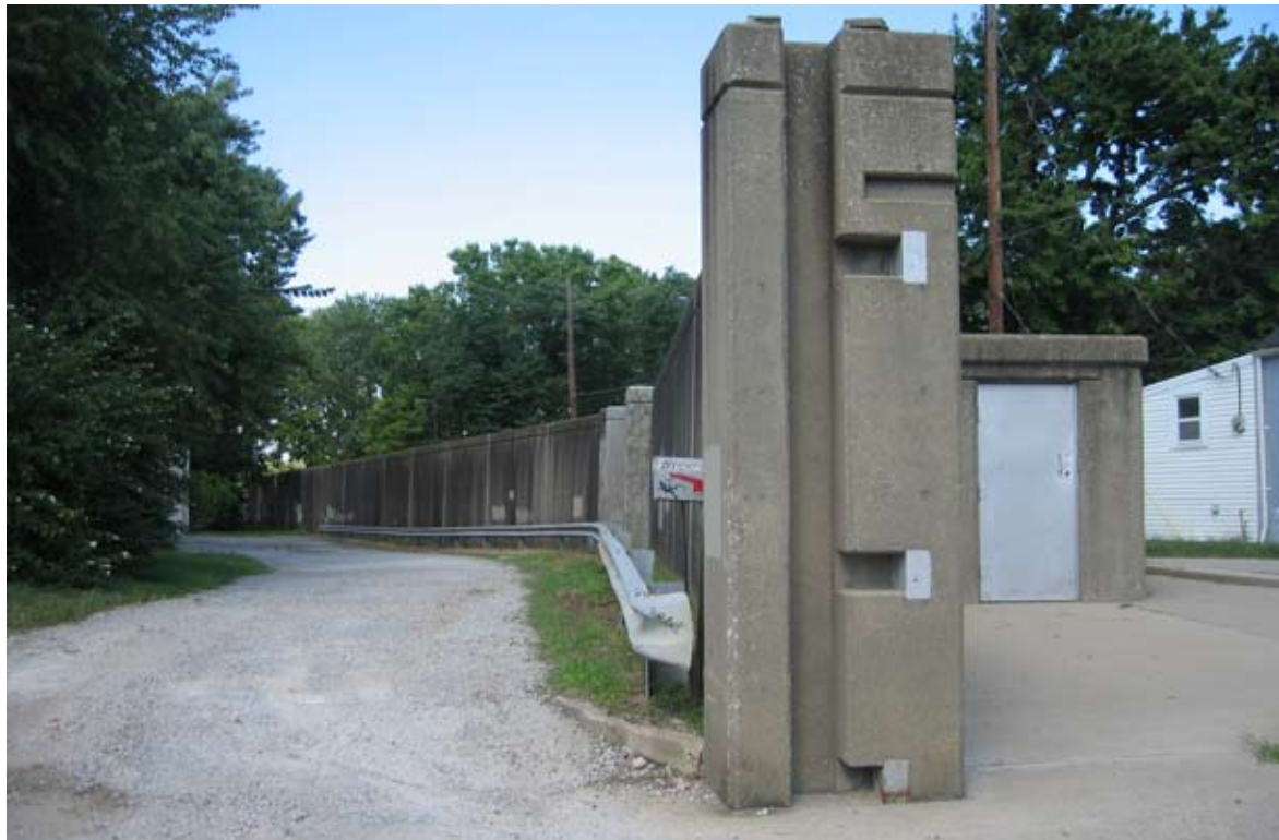
Existing flood walls in Butchertown are approaching 50 years of age and require cribbing at all openings.
